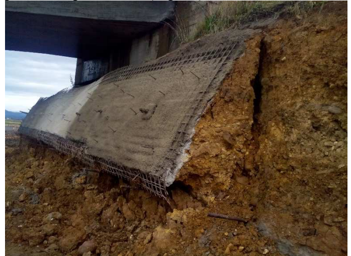
Figure 15. An insufficient observation method can cause more damage than this exemplary little slider
