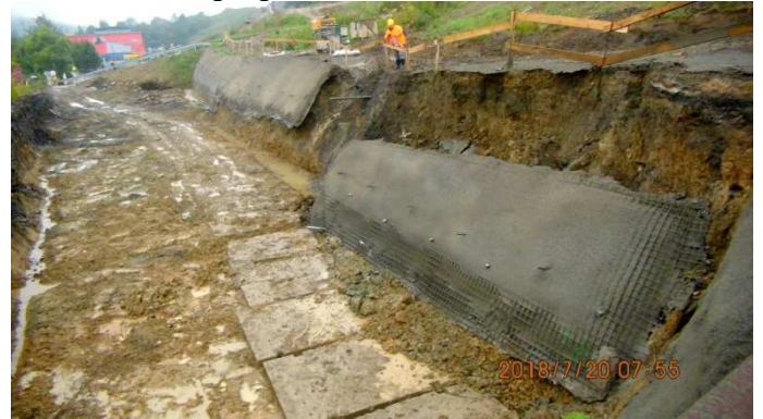
Figure 12. More than a week open unsecured excavation and one-day rain
