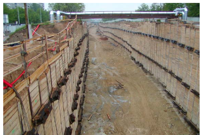
Figure 5 Anchored sheeting walls in the open pit for the cut-and-cover tunnel between Střížkov and Prosek
